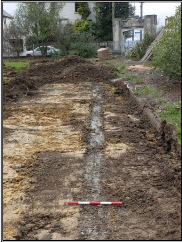
Figure 36 The initial topsoil removal underway on 20 August 2018, revealing the concrete foundations of the 1886 High Street School building just below the surface. The scale is 0.5m long.
