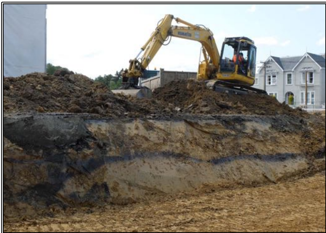
Figure 43 The bulk excavation of the building site underway in March 2019, with the undulating buried soil horizon clearly visible in the bank.
