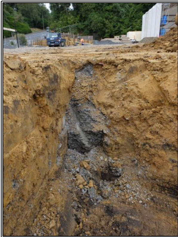
Figure 37 Section cut through the school foundations during bulk excavation of the clay fill on the site, March 2019.
